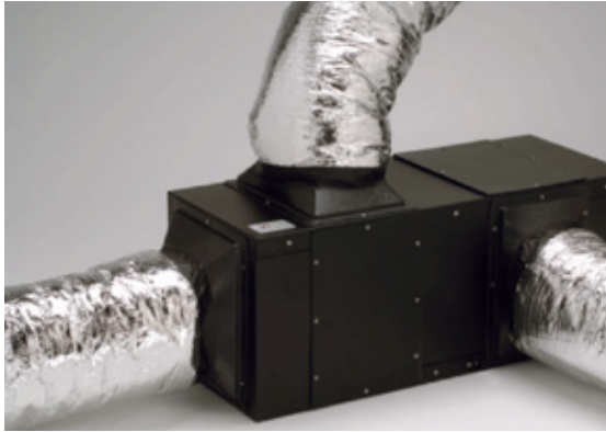
Ducted system with installed duct work
